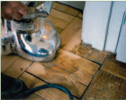
The uneven flooring in the doorway required aggressive sanding. Again, repair was not an option.
