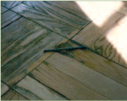
A deep gouge cannot be removed and required filling. Repairing these and similar issues was determined to be too costly.
