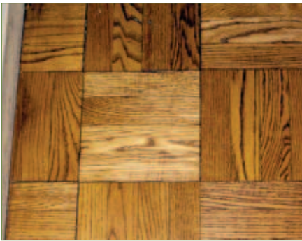
A finished area. Note the cross scratches on the slats and the uneven bevels.
